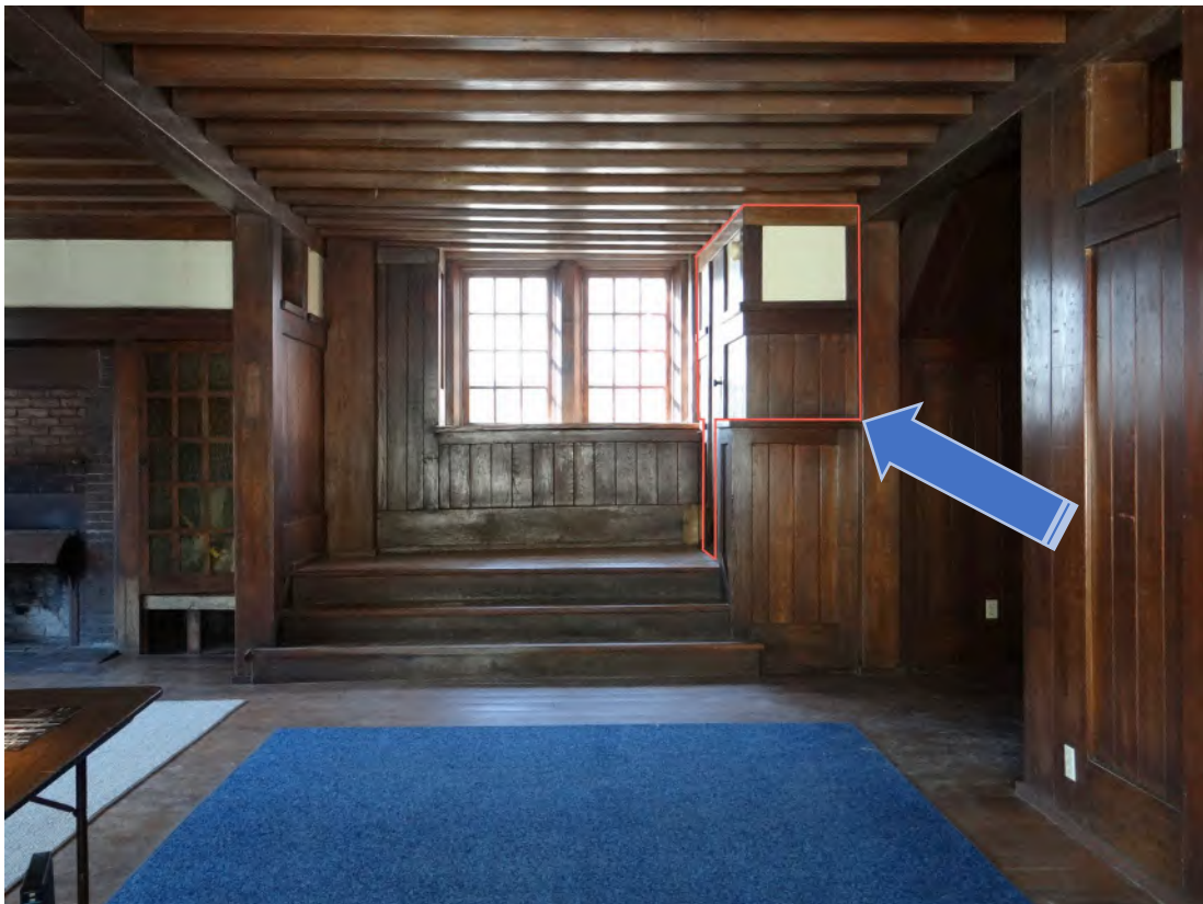
GSH-2 Photo 2 / Stair Hall Looking South. Photo shows the mid-1940s enclosure, outlined in red, built of salvaged chestnut from elsewhere in the house and gypsum wall board. This enclosure was constructed mid-1940s during the Wiles family occupancy. See also Photo 3. 3/15/23, Crawford & Stearns, Architects.
