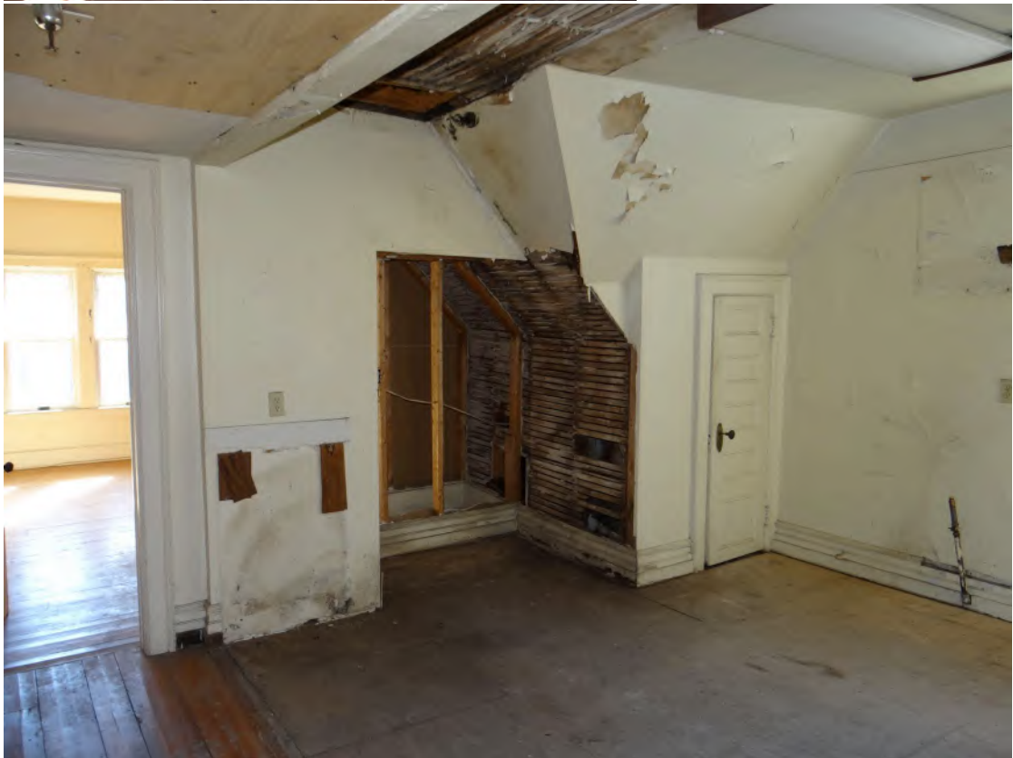
GSH2 Photo 20 / Third Floor – Former Apartment Kitchen. Proposed removals include 1985 plywood floor to allow for examination of historic flooring and framing conditions and removal of 1985 drywall to allow for examination of the roof framing conditions. 2/3/23 / Crawford & Stearns, Architects
