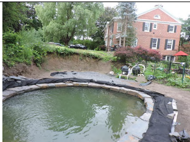
30. Koi pond: inside exiting walls, new waterproof membrane and trim stones. New stacked stone wall at embankment. Center: enclose pool pump in fence.
