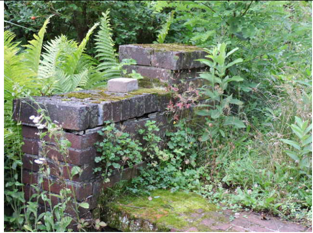
20. Step walls in bad condition.
