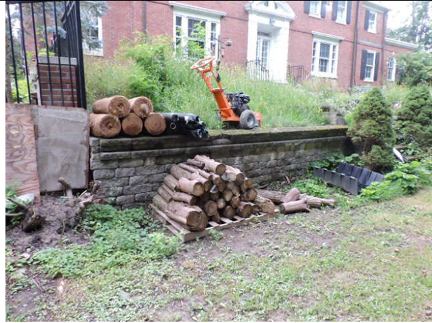
38. Existing concrete wall: covering original brick wall. Remove and repair brick wall.
