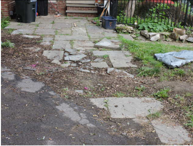
13. Side Entrance Walk: at previous water line replacement replace pavement with new stone.
