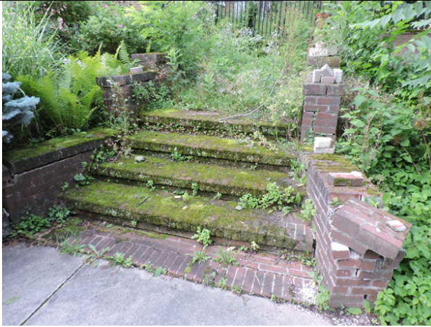
19. Old steps: beyond repair, remove and convert to planting bed behind gazebo.
