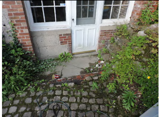
22 Basement door: existing concrete pavers about 12" above bottom of door, frequently floods basement.
