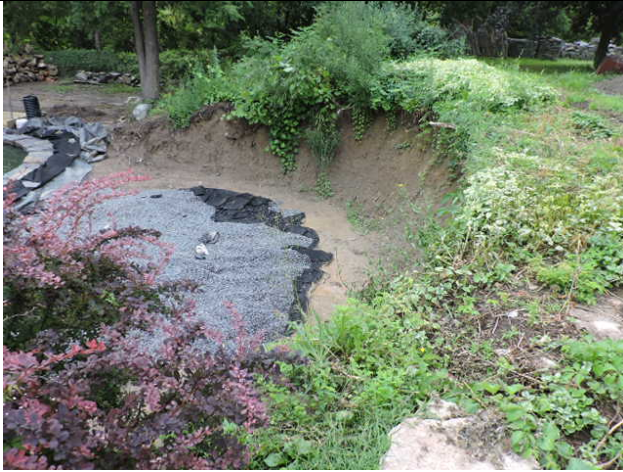
31. Stack stone retaining wall at embankment, new blue stone paving around koi pond.
