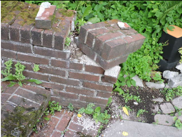
21. Steps and wall in bad condition.
