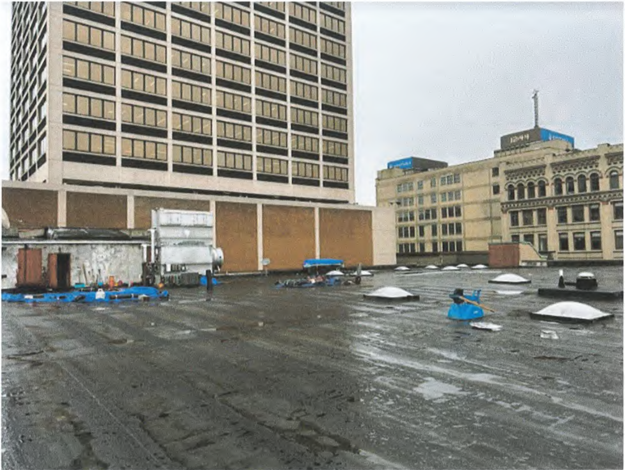
Photo 7) Looking Southwest from the Salina front corner of the roof. In the picture are the two existing staircases that will service the future restaurant. A third will be extended to provide proper egress.
