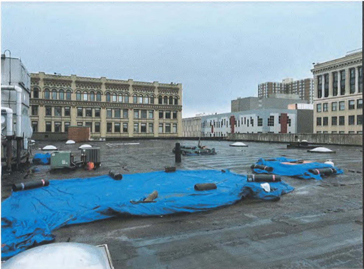
Photo 6) New Roof currently being installed in prep of the rooftop restaurant. On the roof facing Southeast. The restaurant will take the front half of the roof.
