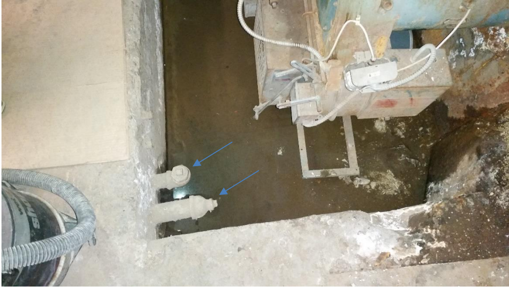
View of the former fuel oil supply and return piping at the boiler.
