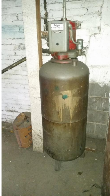
View of the hydraulic loading dock tank.
