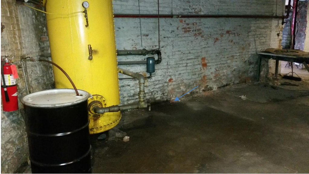
View of oil floor staining at a former air compressor.
