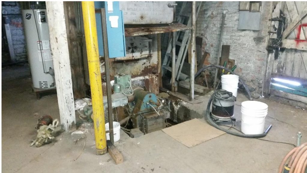
View of the boiler.
