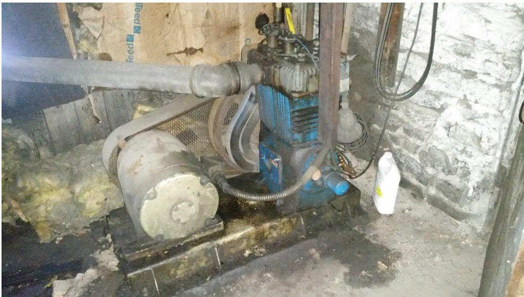
View of oil floor staining at an existing air compressor.
