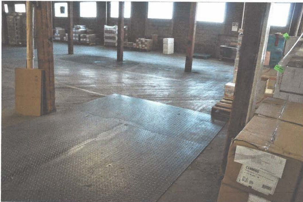
F-8 3rd FLOOR—Wood strip flooring with rubber traffic surface—Note: Wood strip flooring is in poor condition with warping and deterioration of the surface and along the joints.
