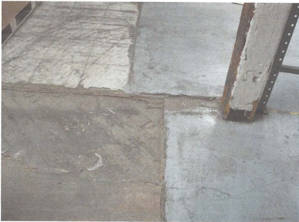
F-7 3rd FLOOR— Detail of the original strip wood flooring with a plywood overlay and VAT and Painted Cementitious Traffic Surface
