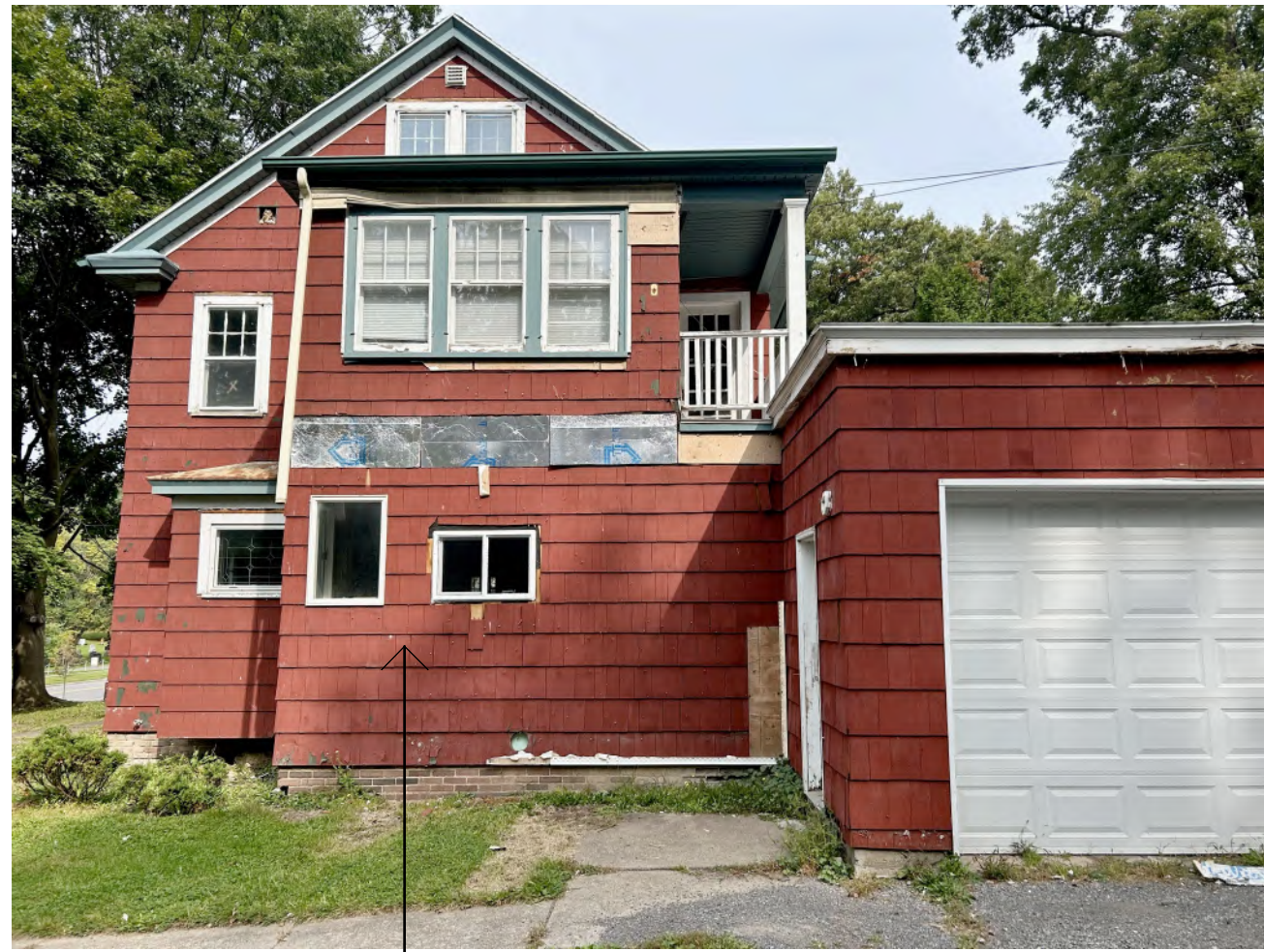
MISC VINYL WINDOWS CASEMENT/SLDG, RECENTLY ADDED NOT ORIGINAL, DH REMOVED IN PREVIOUS REMODEL WITH ACCESS DOOR TO KITCHEN SPACE.
