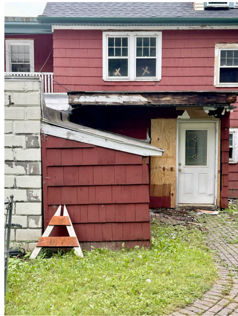
ROTTED ONE STORY WING ROOF. REPLACE WITH HIP ROOF AND FRAMING. GARAGE AND SHED TO BE REMOVED
