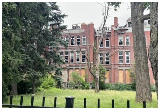
June 2025 photo following the March fire. (Office of the City Auditor)
