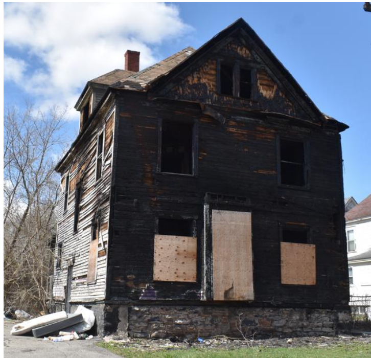
March 2025. Property remains standing heavily damaged (Office of the City Auditor)
