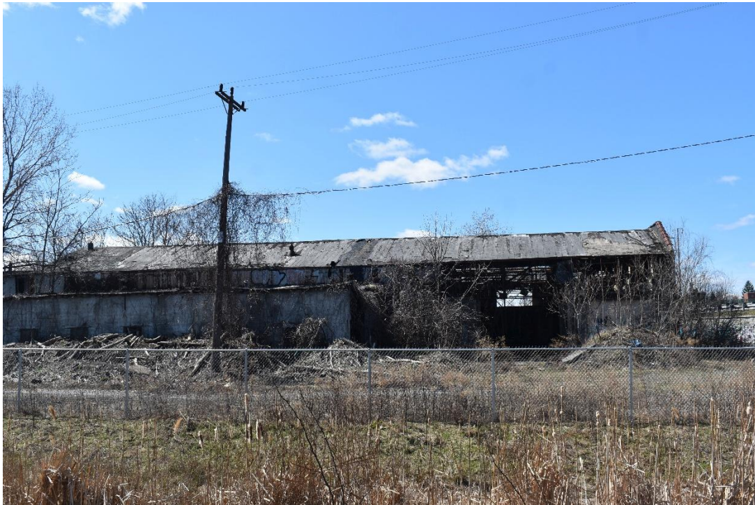
March 2025. The building remains vacant and deteriorating following fire. (Office of the City Auditor)
