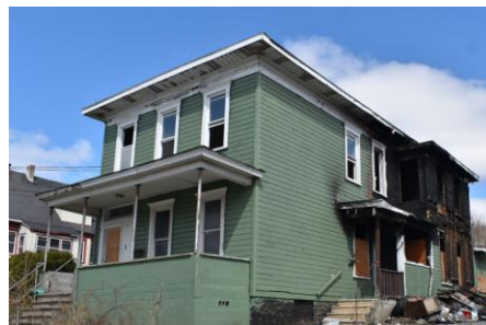
March 2025. Rear of property shows significant fire damage. (Office of the City Auditor)
