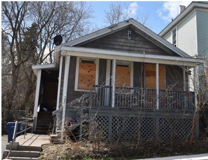
March 2025. Property still boarded after fire damage. (Office of the City Auditor)
