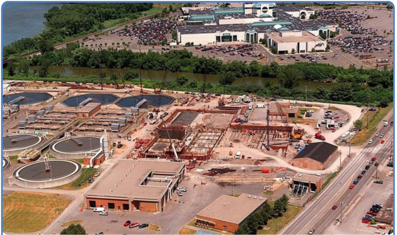
Syracuse Metropolitan Wastewater Treatment Plant
