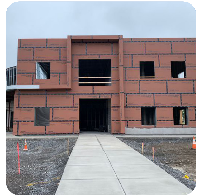
Montreal Construction transformed an old truck terminal at 1004-1014 N. Geddes St. in Syracuse into modern office space.
