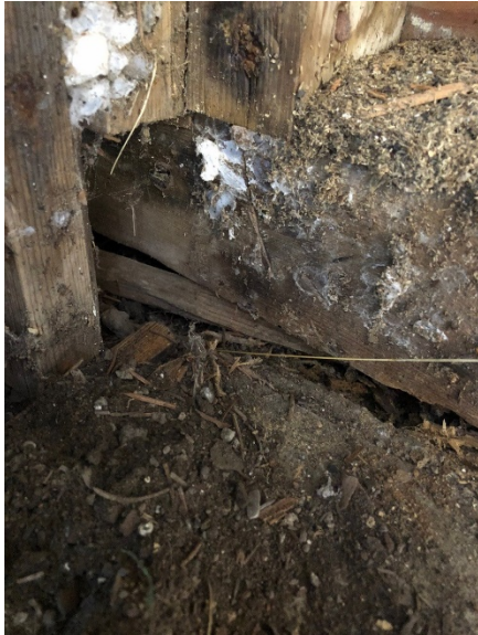
PHOTO #3 – Deteriorated sill plate, cantilevered & not in contact with the foundation. Further portions of the sill plate sitting on dirt.
