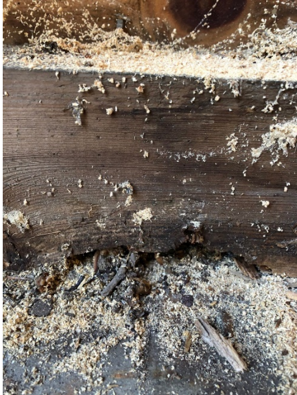
PHOTO #2 – Deteriorated sill plate.
